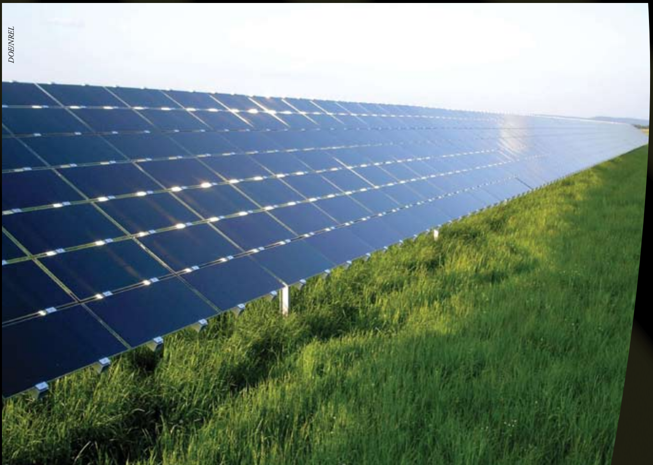
A 1.45-megawatt thin-film solar park in Germany operated by Beck Energy.
